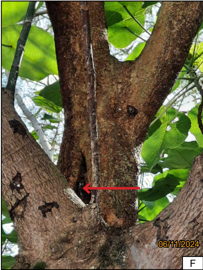
T2 (DEFECT A)
