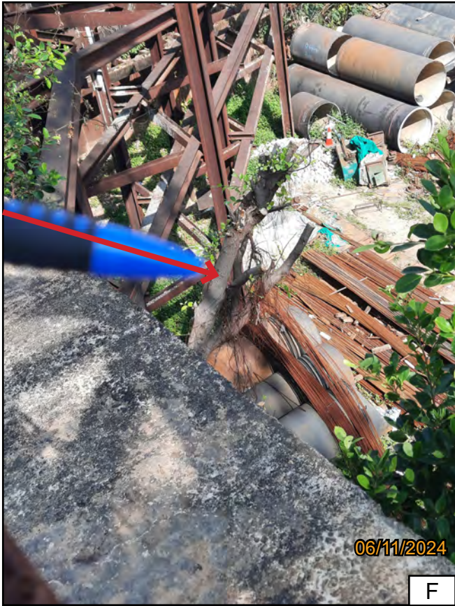
T10 (DEFECT A)
